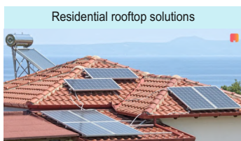
Residential rooftop solutions
