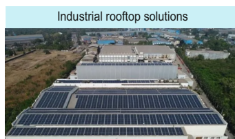
Industrial rooftop solutions
